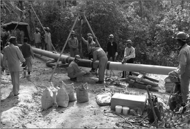
The laying of a gas pipeline directly through Lawachara National Park in 2005. Controversy over the issue stimulated a more active early development of the Lawachara Co-Management Committee. [Philip J. DeCosse]
