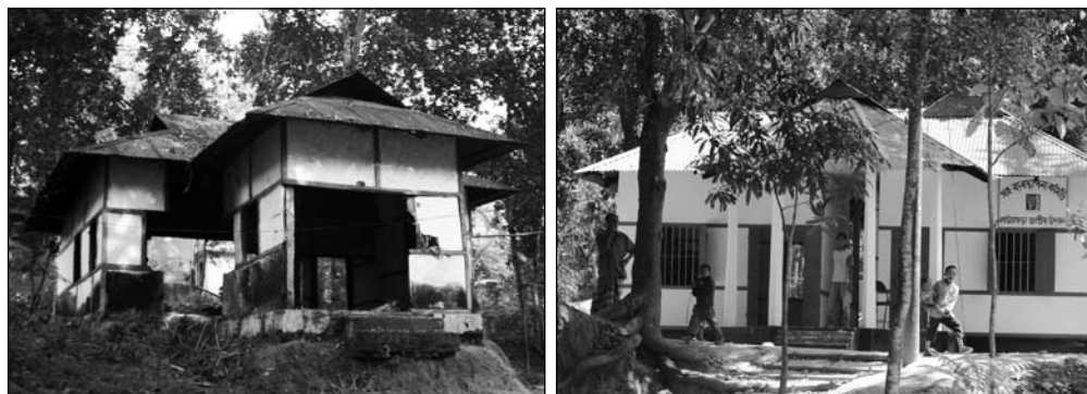
The Co-Management Organization office at the Lawachara National Park looks like a newly constructed building in comparison to its previous condition where it had broken windows, discolored walls and dirt all around. [Abu Syed Samiul Islam]
