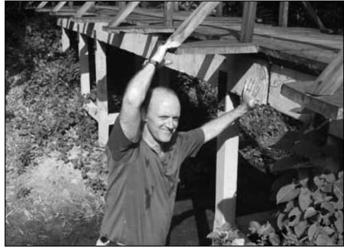
Following the Vitti guidelines, the newly constructed bridge proved to be more stable and safer. [Md. Modinul Ahsan]
