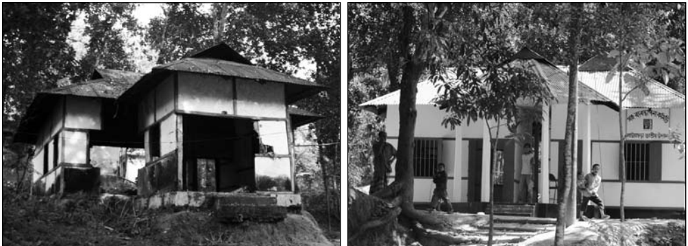
The Co-Management Organization office at the Lawachara National Park looks like a newly constructed building in comparison to its previous condition where it had broken windows, discolored walls and dirt all around. [Abu Syed Samiul Islam]
