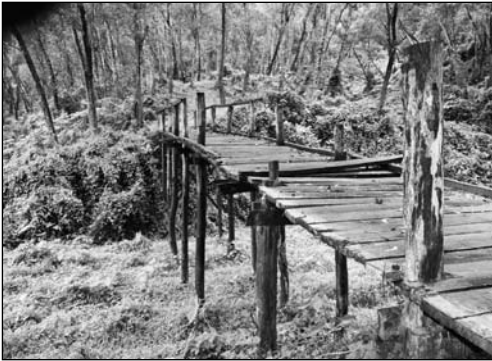
The old bridge which was built without following proper guidelines was unstable and dangerous for visitors. [Quamrul Ahsan]
